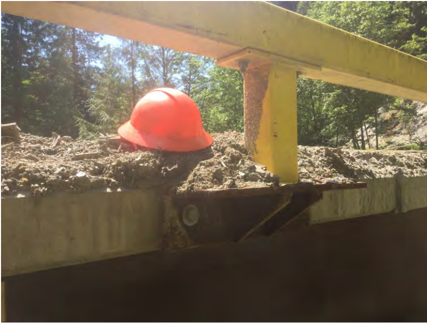
Amount of sediment on deck
